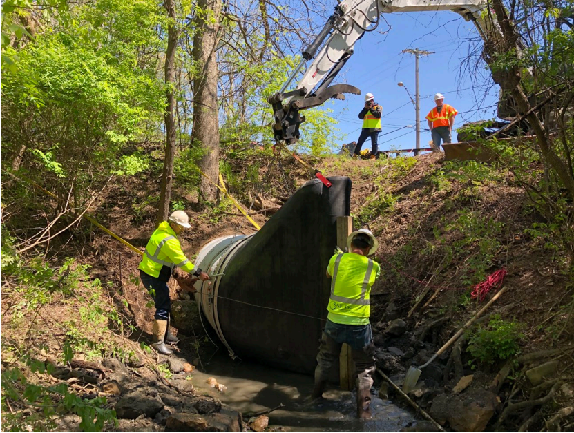
Figure 30. U.S. Army Corps of Engineers Buffalo District Contractors Install a Check Valve at Wolf Creek as Part of the Ohio-Erie Canal Aquatic Nuisance Species Project in Akron, Ohio
