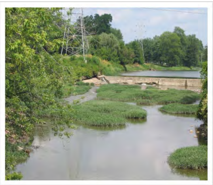
Photo showing Huntington Dam. Damage can be seen on the left of the dam but currently serves as an adequate barrier against fish movement.
