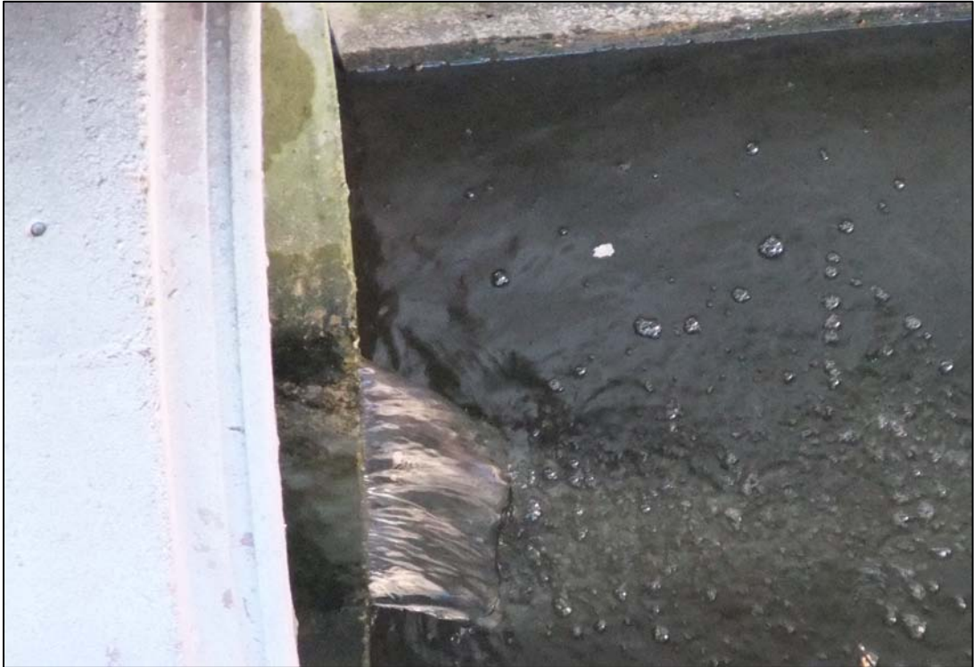
Exhibit 4. Observed water flow from outfall after flush
